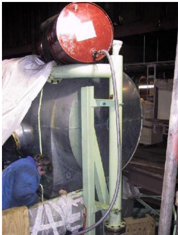
Additional lubrication oil tank connected to the fuel rail to keep it under constant static pressure.
