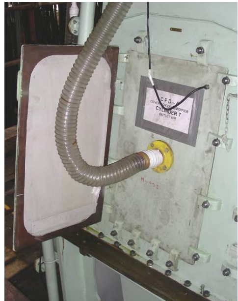
Dehumidifier outlet air taken from the crankcase
