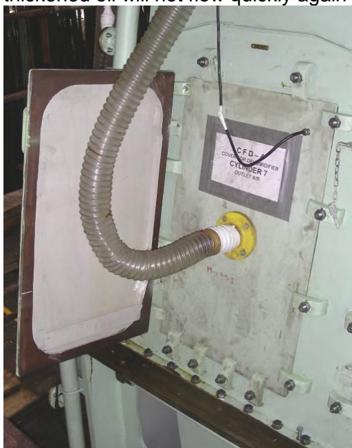
Sample of hose connection of dehumidifier system.
