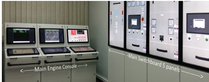
Example of W-Xpert Full Mission Simulator (FMS) arrangement: the 'Engine Control Room' with Main Switchboard and Engine Console
